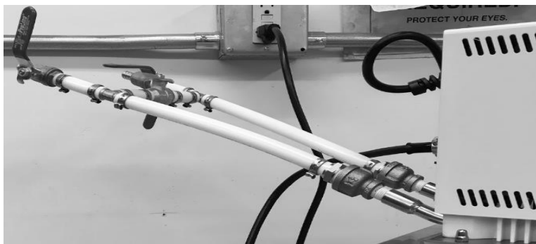
Figure 6. Bypass loop with three ball valves.
