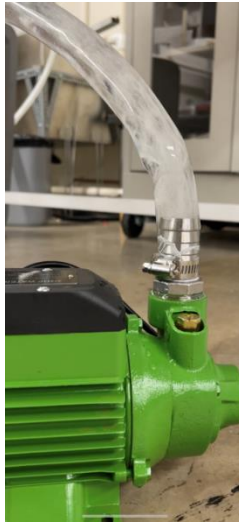
Figure 10. Bubbles at the outlet of the pump.
